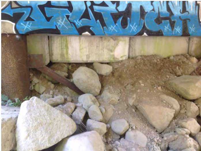
lock blocks under left cap differential settling
