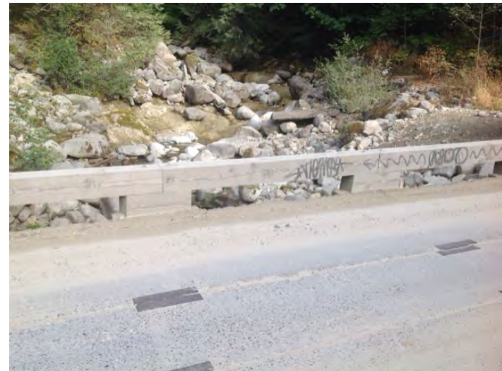
upstream guardrail new
