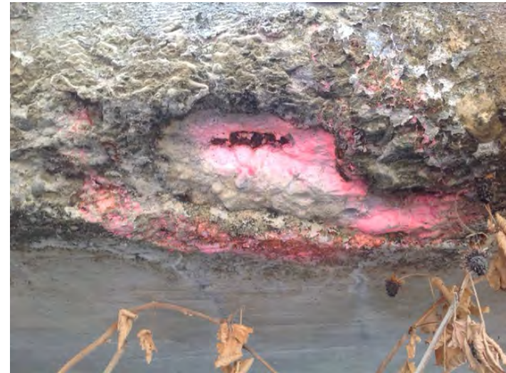
spalling concrete and corroding rebar
