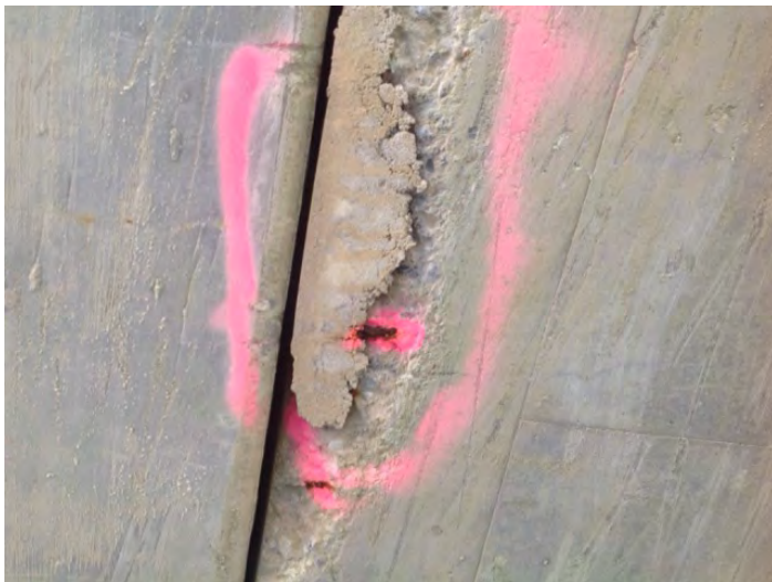
spalling concrete and corroding rebar
